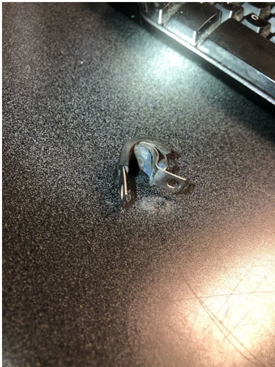
Picture 3 – Deteriorated clamp
