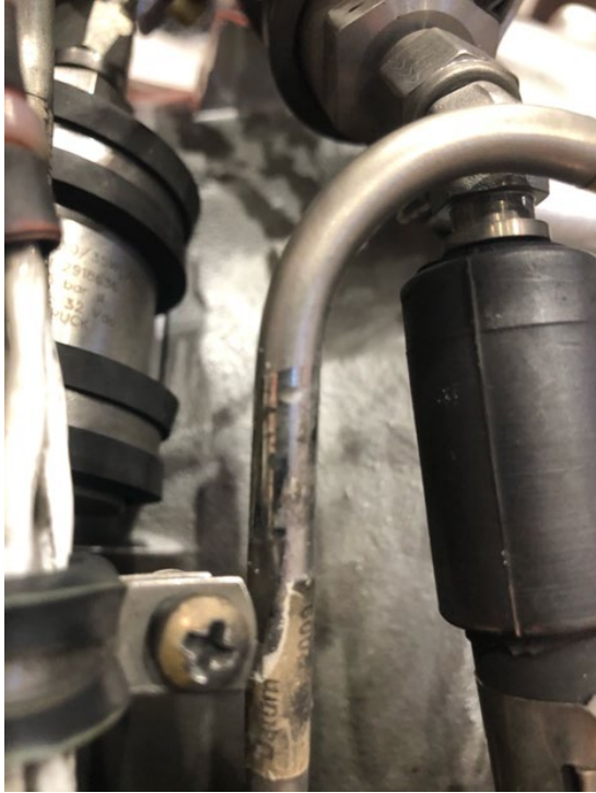
Picture 2 – Clear damage caused to oil tube by clamp
