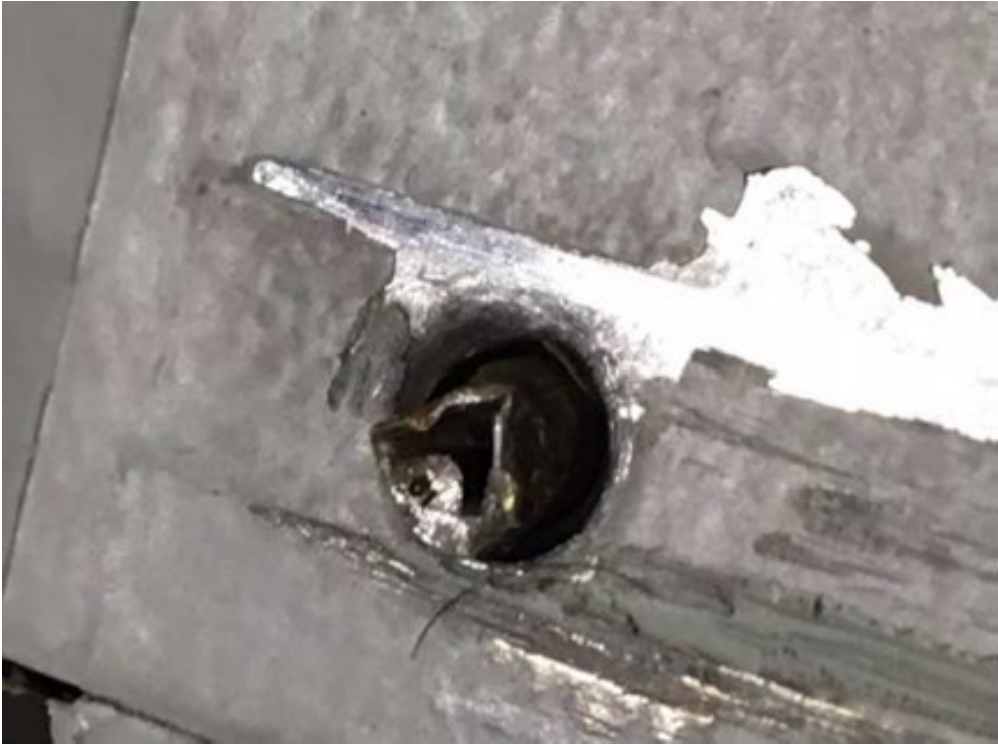
Figure 4: Damaged screw head missing
