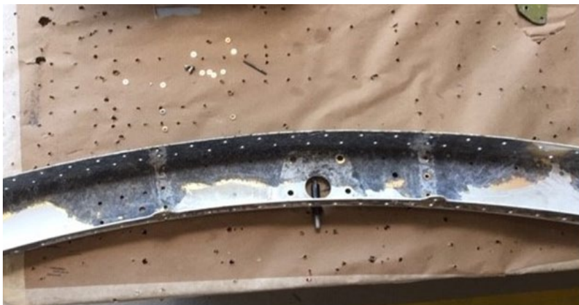
Figure 2: Frame showing corroded area
