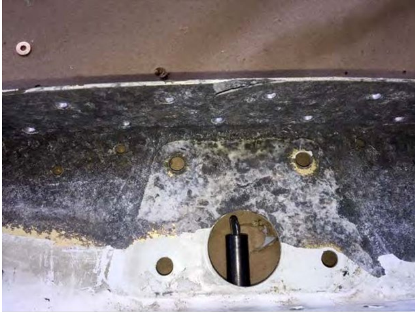
Figure 3: Close-up of corrosion
