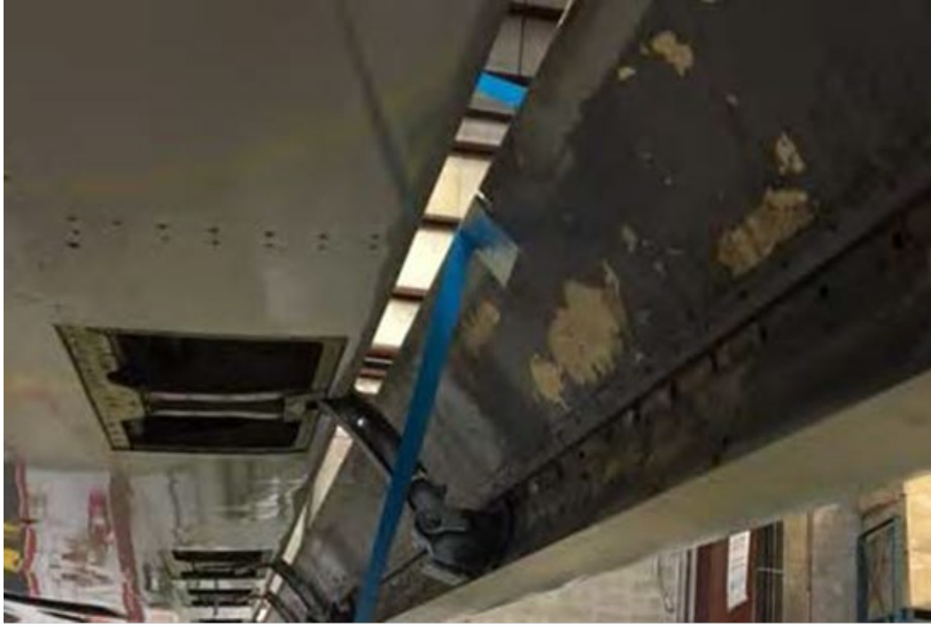
Figure 1: Slat showing location of damage in trailing edge
