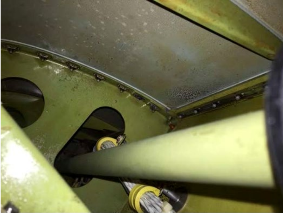
Figure 3: Underside showing anchor nuts
