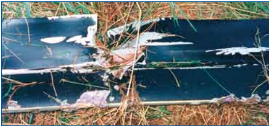
Section of main rotor blade showing chain strike marks on leading edge.
